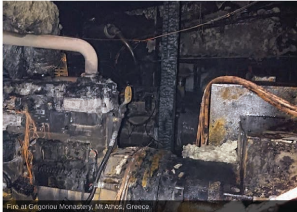
Image: Damaged electromechanical equipment after the Grigoriou Fire
